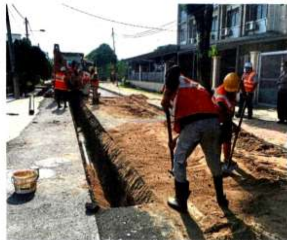
Air Selangor's pipe replacement project in Sections 1 and 2, Petaling Jaya, is scheduled to be completed by end of the year.
